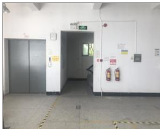
Photo of fire safety equipment Exit sign and emergency light and fire alarm.JPG
