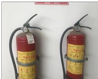
Photo of fire safety equipment Fire extinguishers.JPG
