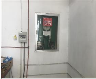
Photo of fire safety equipment Fire hydrant.JPG
